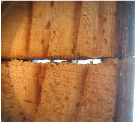
Fig. 7: Crack in Glue Line and Seal
