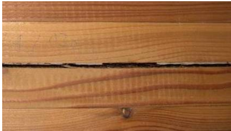
Fig. 8: Crack in formerly sealed Glue Line
